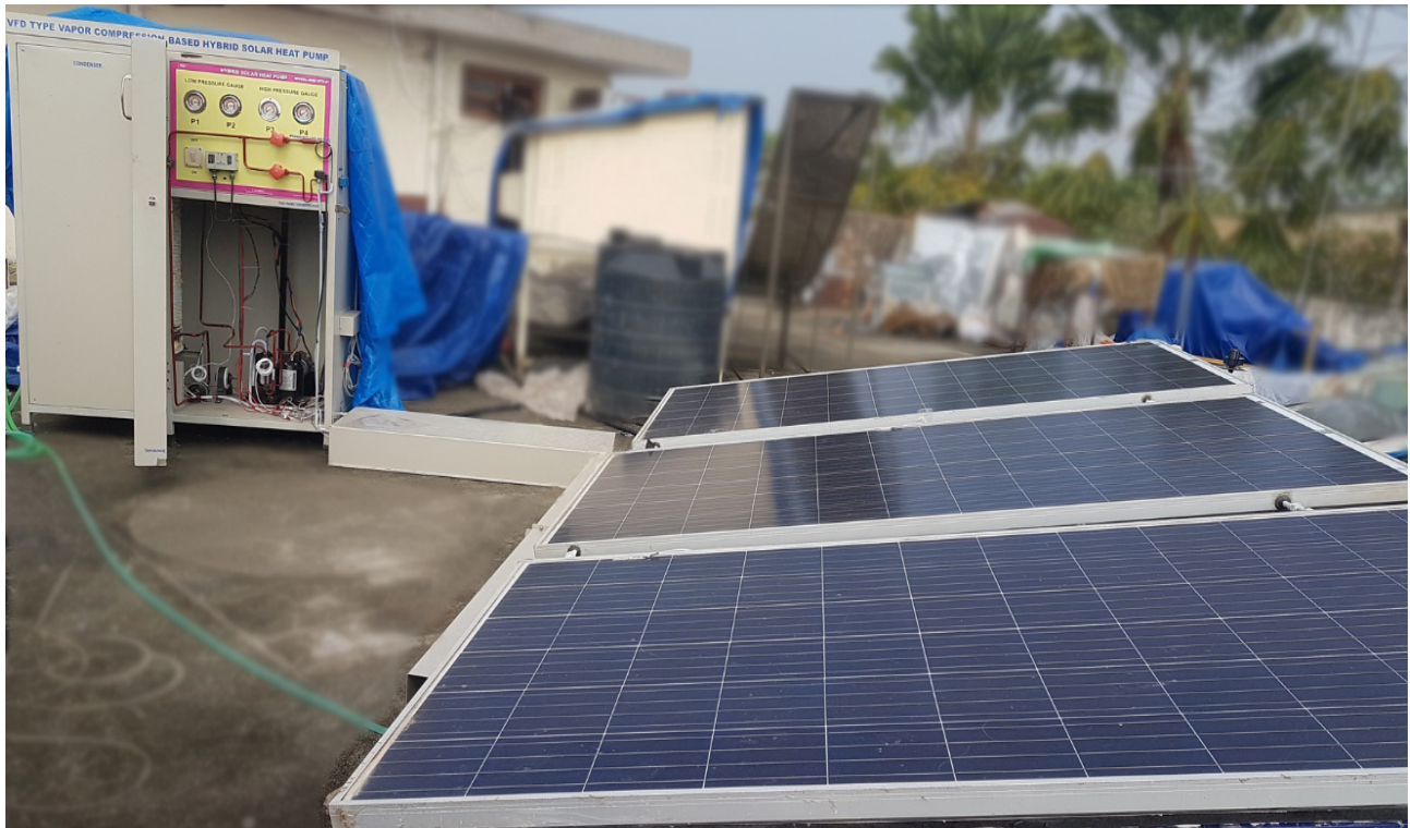
Figure 2 – Photographic view of the heat pump-based PV-T water heater system installed at the SEC
