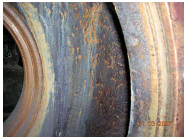
Figure 2 – Cavitation of the helix after a year of operation of the pump.
